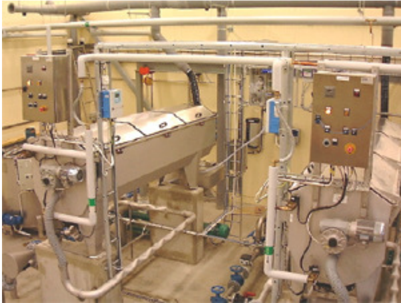
Two drum thickeners Siljan RotoMaster SF 17 installed before a digester
