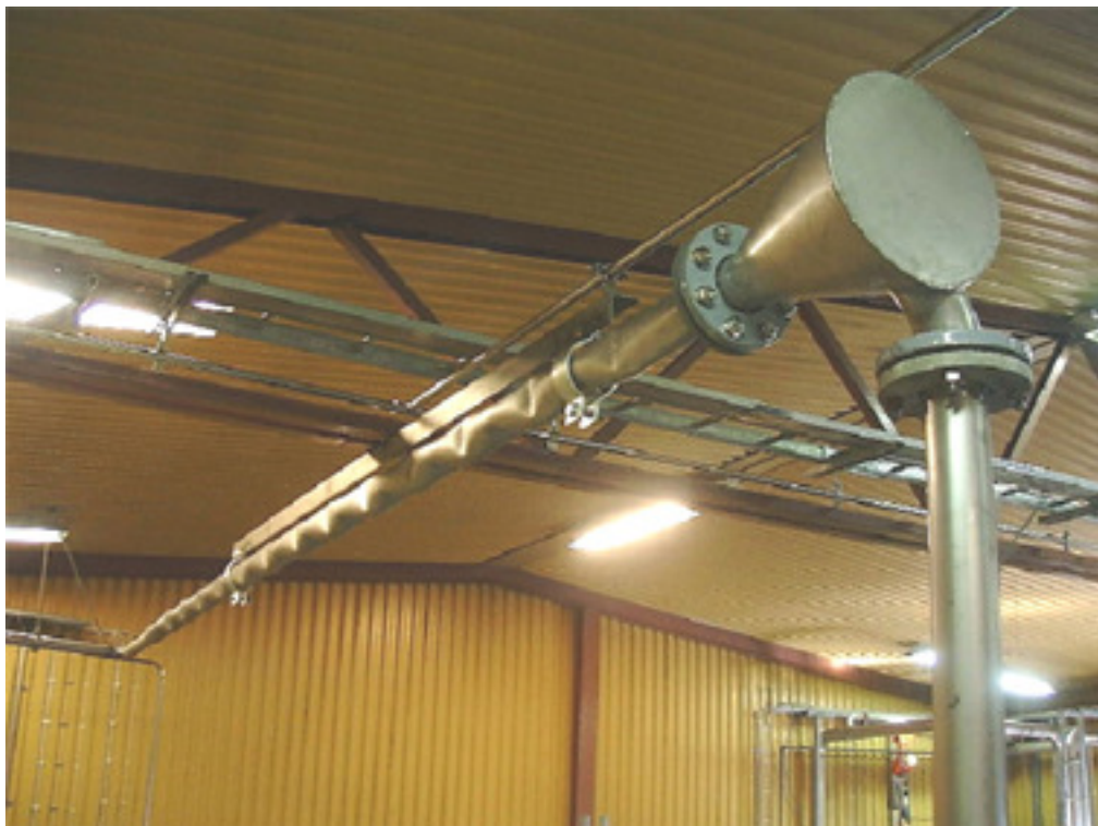
Conical mixer and static tubular mixer have been installed above the SF 3 thickener, to save space.
