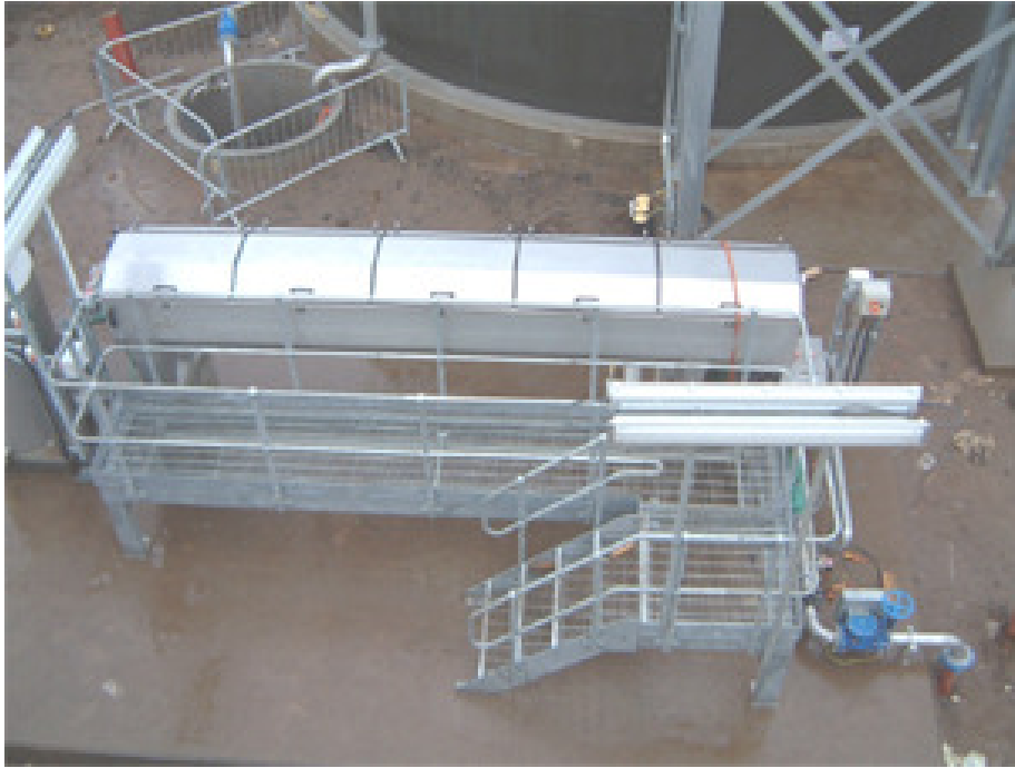
One drum thickener Siljan RotoMaster SF 35, at site in Bonnybridge, Scotland.
