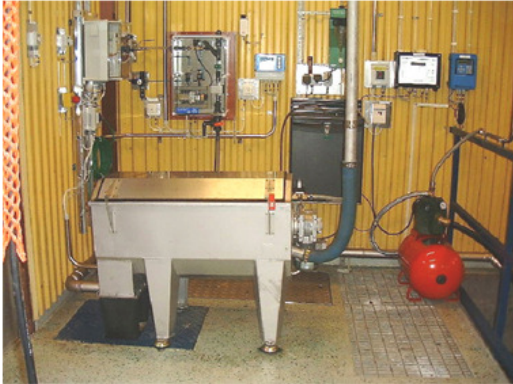
A Siljan RotoMaster SF 3 (the smallest machine, 3 cbm/h) installed in a small WWTP in the middle part of Sweden; On the wall the Siljan Polysave unit, which minimizes the need for attention of the operator, makes 24 hours operation more reliable and saves expensive polymer.
