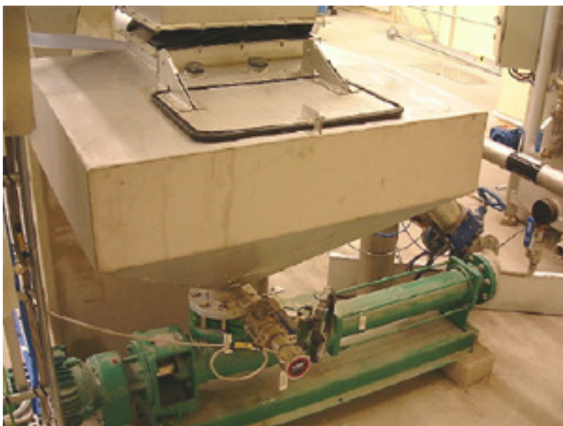
Sludge hopper with level transmitters, after the drum thickener, connected to the pump for thickened sludge
