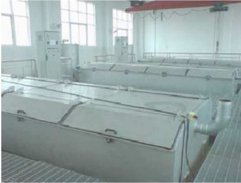
3 x Siljan RotoMaster SF 120 drum thickeners installed in the Louyang Chandong WWTP, in China.
