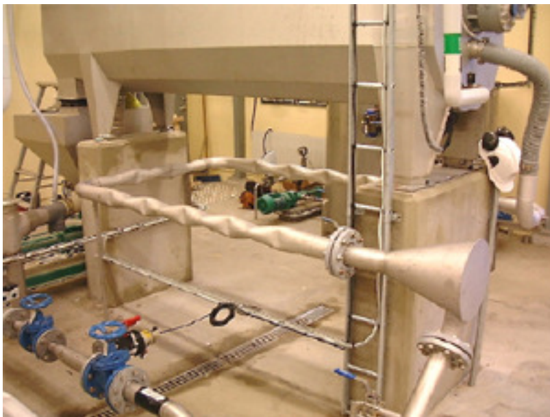
Conical and tubular mixers for mixing and flocculation before sludge thickening
