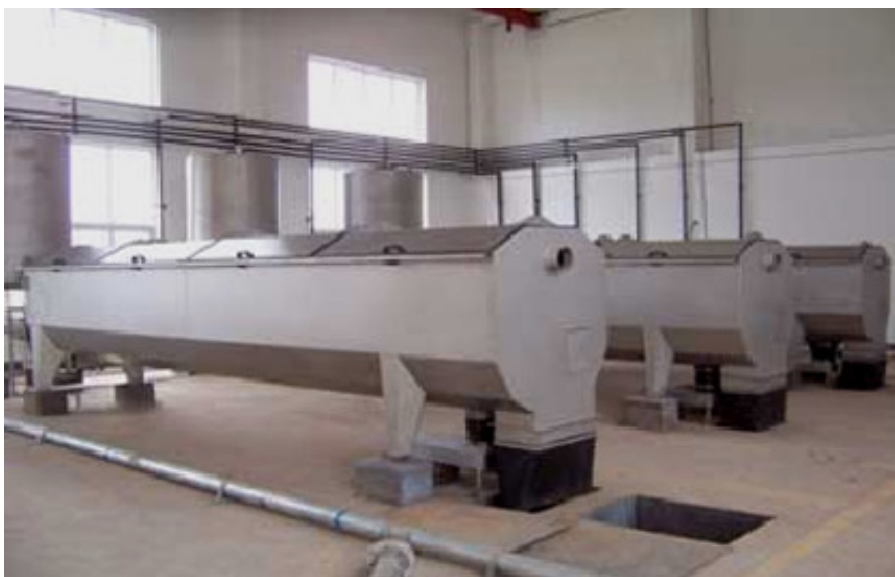
3 x Siljan RotoMaster SF 60 drum thickeners installed in the ZhuZhou WWTP in Hunan, China
